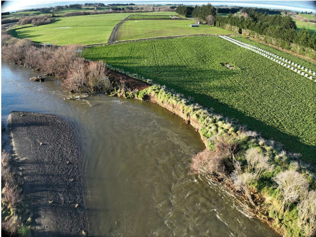
Erosion of the True Right Stopbank below Otautau
