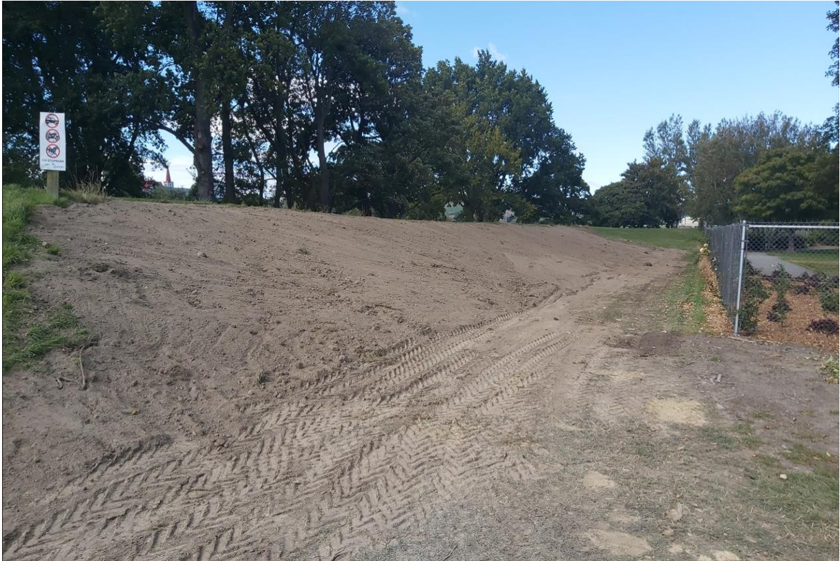
Finished result after stumps removed and repairs made to Stop Bank at Richmond Street Gore
