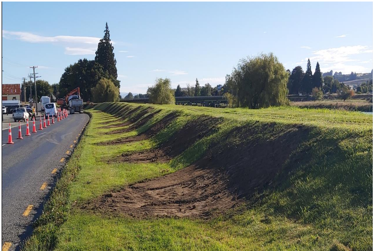
Finished result after repair work carried out along River Street at Gore
