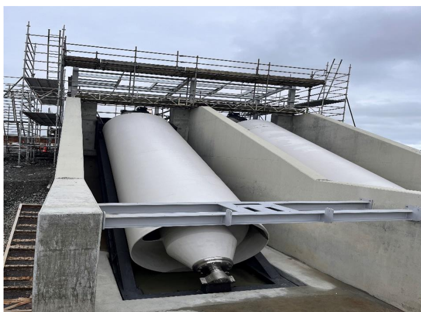
Stead Street pumps installed
