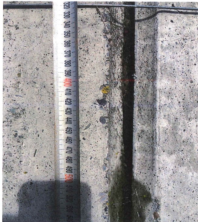
Closeup view of level of damp concrete below top of pond.
