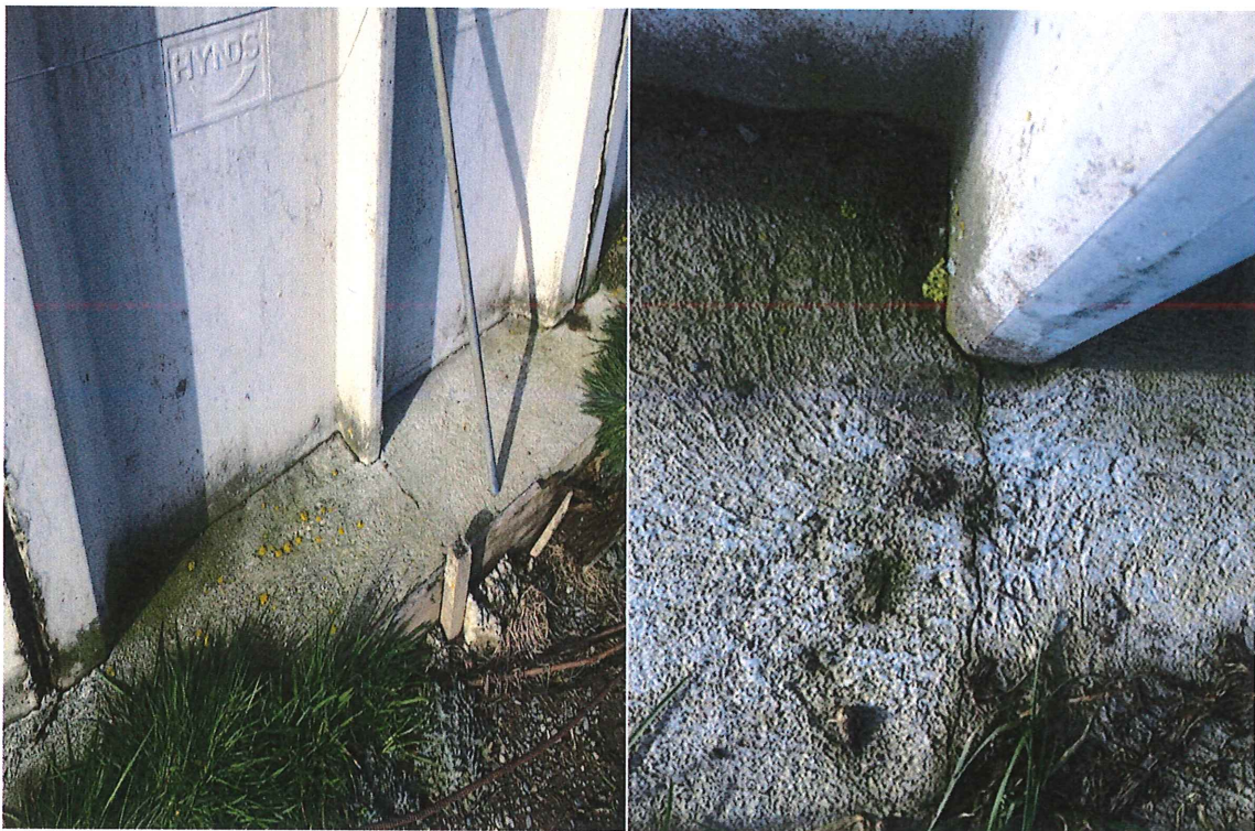
Typical view of ground level ring beam and close up view in RH photo of typical shrinkage crack initiated at smaller centre panel rib.
