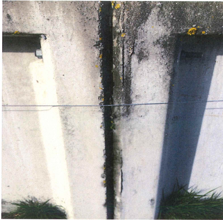
External view of previous top joint showing sealant in good condition and minor damp concrete at the lower level.
