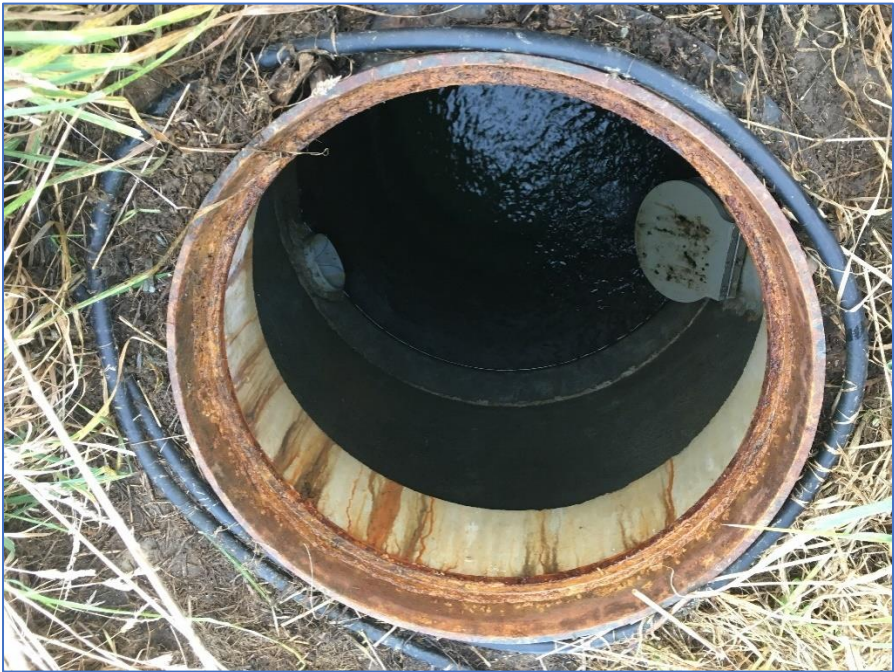
Figure 5: Leak detection port with no trace of effluent
