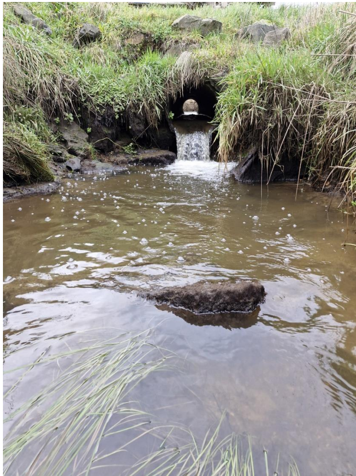
Figure A4: Perched culvert to be remediated at proposed tributary enhancement site.
