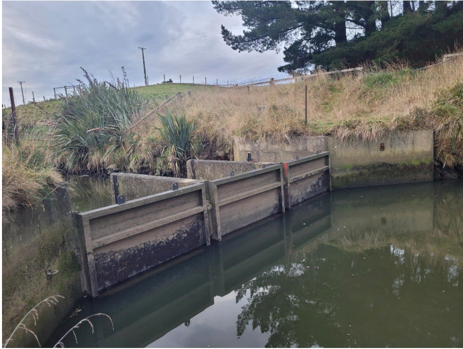
Figure 2 Photo of Titiria tide gates, close to high tide, taken on a site visit on 10th August 2024, standing on true right bank of diversion channel, downstream of the tide gates
