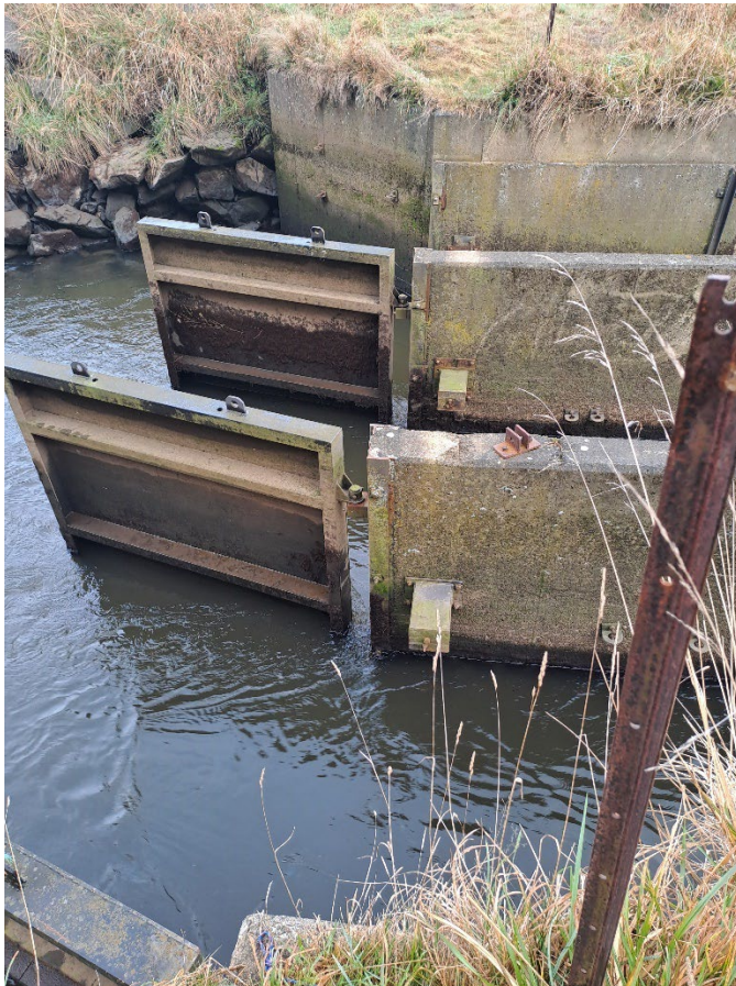
Figure 3 Photo of Titiria tide gates, close to low tide, taken on a site visit on 10th August 2024, looking across the diversion channel while standing on the true left bank
