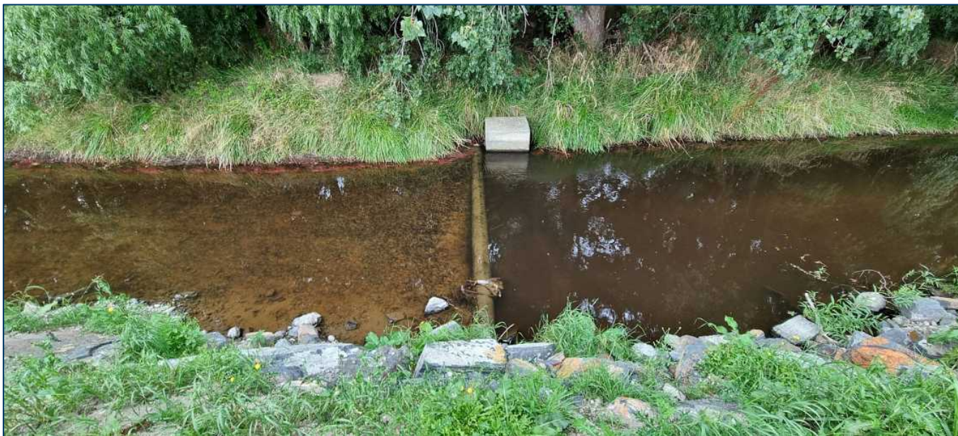
Figure 1 Diffuser in Winton Stream replacing six individual discharge pipes
