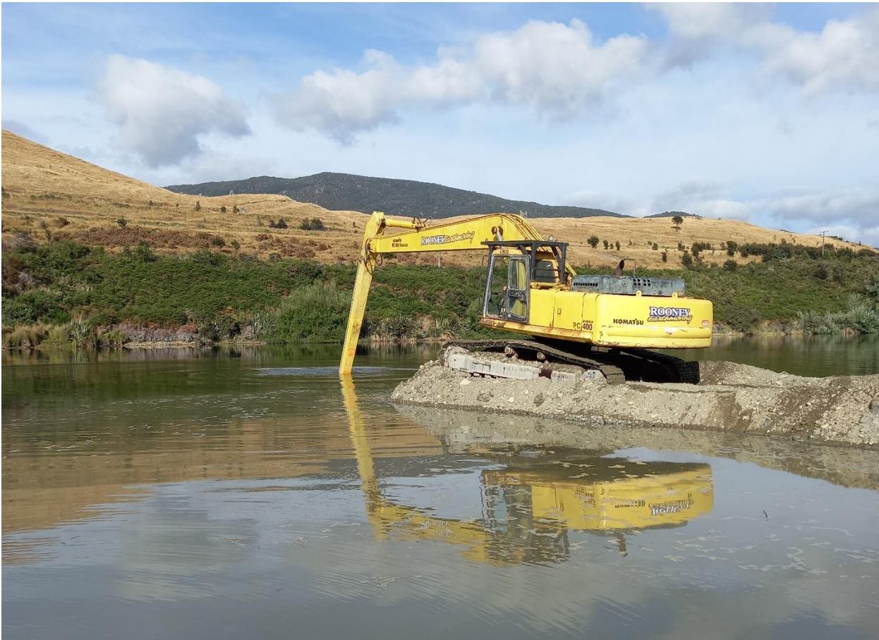
Figure 5.3: 40t long-reach excavator, excavating trial hole at Location A from constructed gravel bund.
