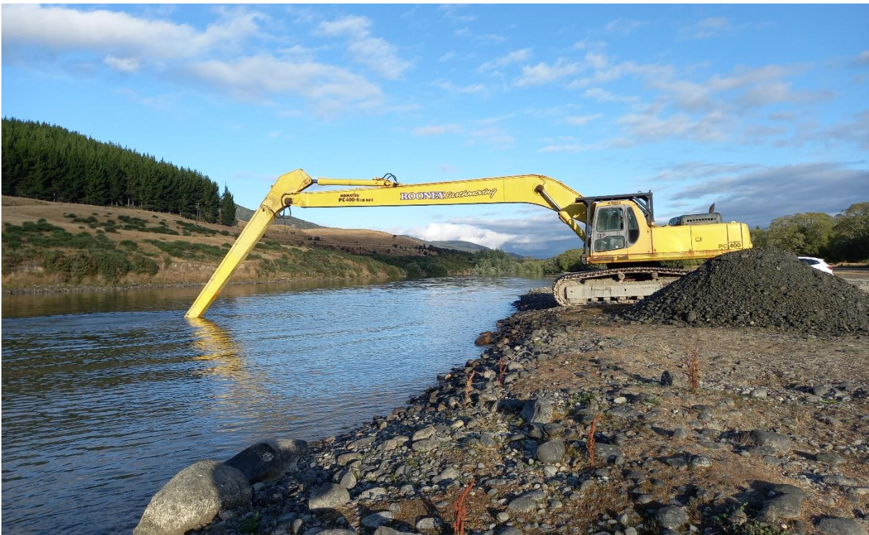
Figure 5.4: 40t long-reach excavator, excavating trial hole at Location D from riverbank, with pile of excavated gravels adjacent.
